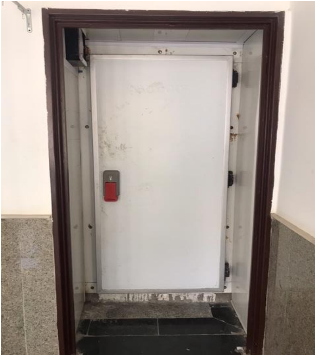
Cold room (Y
